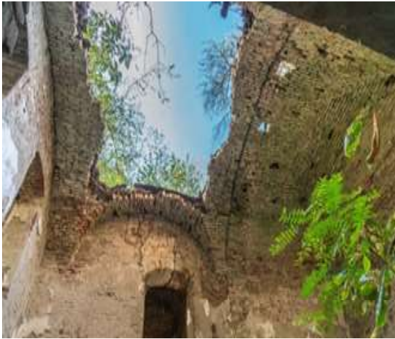
Fig. 8. Completely collapsed vault in the sanctuary
