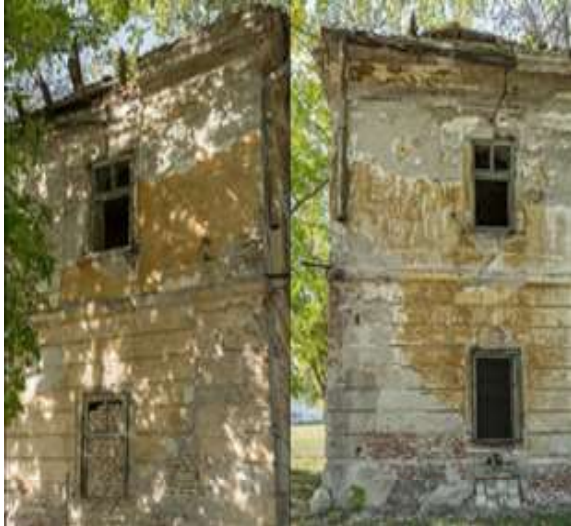
Fig. 3. Vertical cracks at the corner of the building
