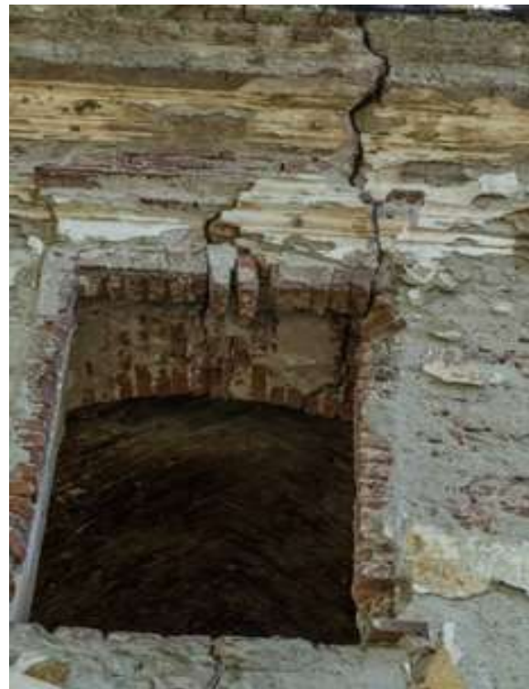
Fig. 5. Cracks in the spandrel beams
