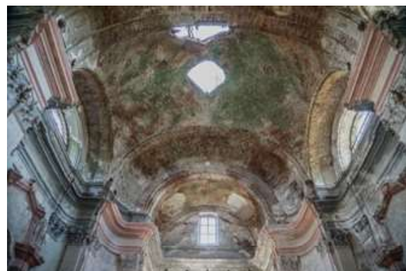
Fig. 7. Partially collapsed vault in the church
