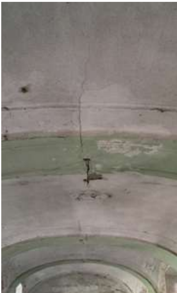
Fig. 4. Cracks in the arches and vaults
