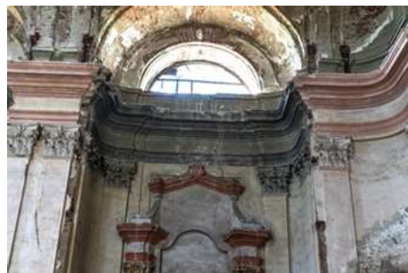
Fig. 6. Cracks in the monastery walls
