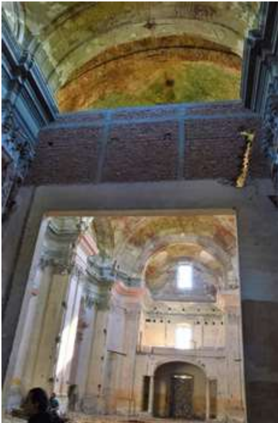
Fig. 9. Unauthorized masonry wall with RC frame
