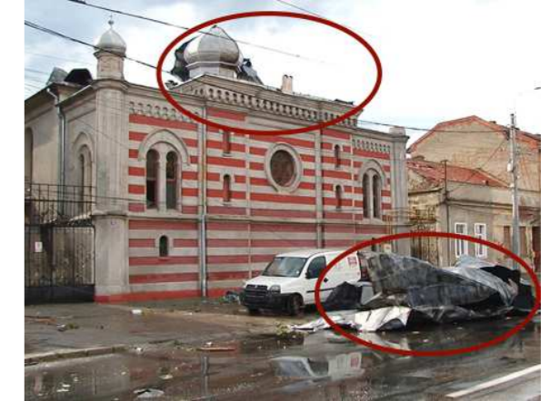
Fig. 7. Roof structure damaged by wind ([14])
